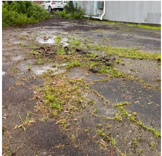
Photo 8 Pavement condition at rear of site
